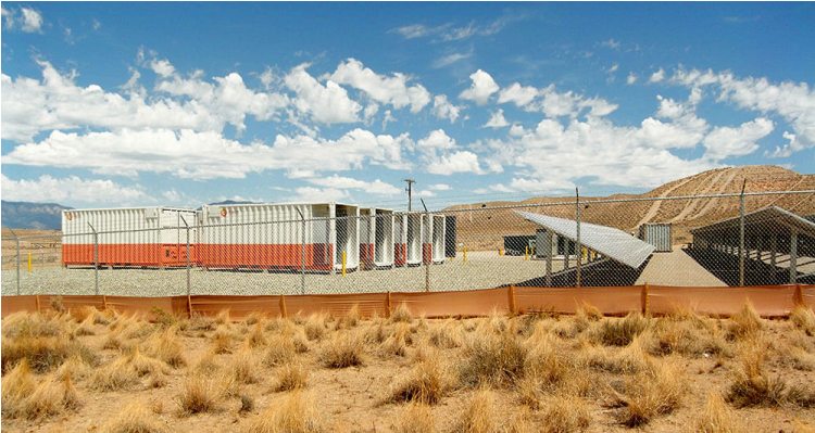
PNM's Prosperity Energy Storage Project
